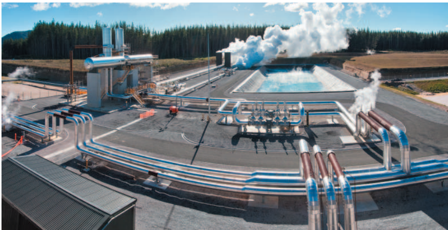
HERA member Mighty River Power's Ngatamariki power station will increase the company's geothermal generation to more than 40% of capacity
